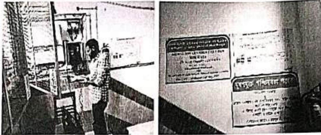
Figure 8 Measurement of Solar PV Generation at 10 kVA Inverter LT Panel-1 (West Side)
